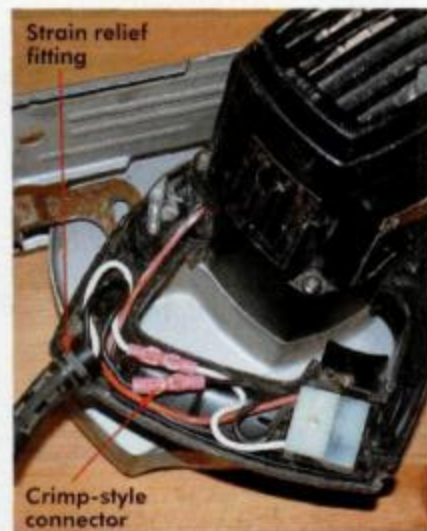
New cord installed
