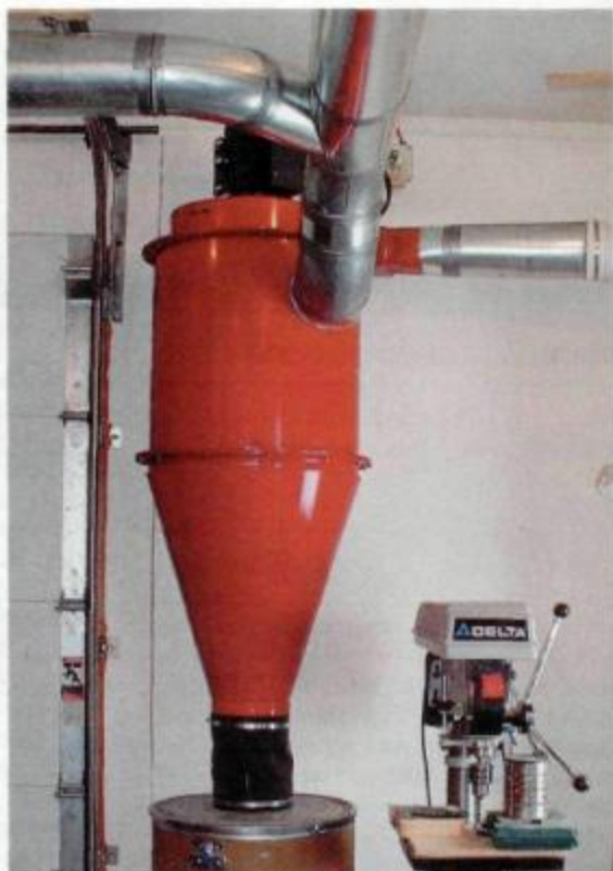
Installed cyclone system
